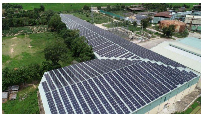
Rooftop solar power system of SBT at TTC Gia Lai
